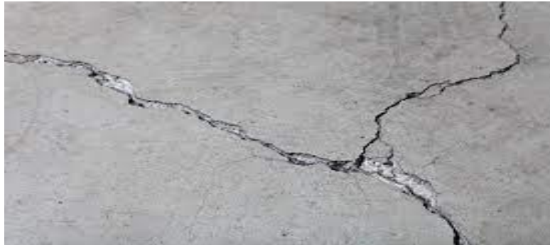
Figure 4. Cracks in slab
