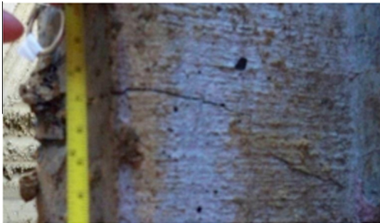
Fig. 18. A flexural crack found at a depth of 2.74 m below the top of P4.
