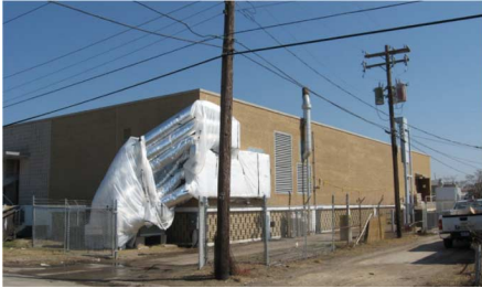
Fig. 12. AT&T's Sherwood CO after Hurricane Ike.
